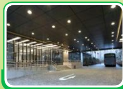
Large Area Lighting
